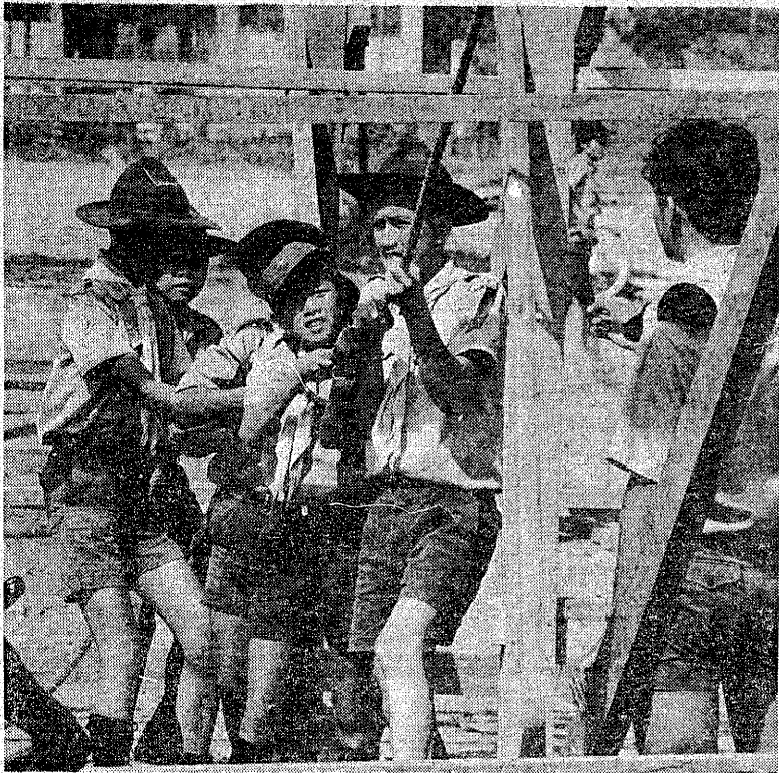
Vietnamese Boy Scouts haul on a rope to pull up a pre-fab frame at the Petrus Ky housing area in Cholon, a Saigon suburb, where a semi-permanent refugee camp is rising.
